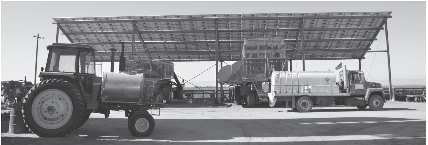
The solar-powered irrigation pumping system array on Gary and Mari Martin’s farm.
