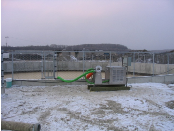
SAR™ Aerator at Rol-Land Farms Lagoon
