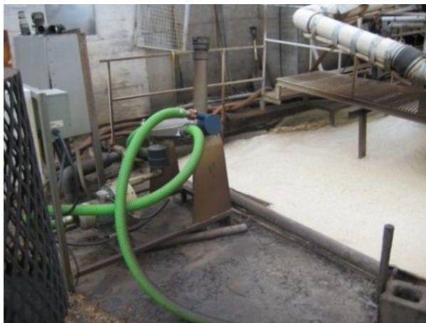
SAR Aerator producing the Froth Layer
