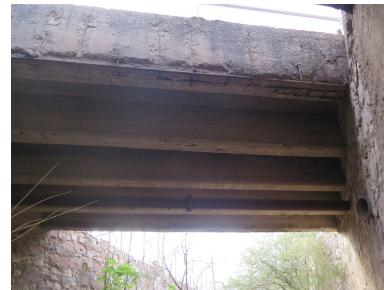
Condition of the bridge girders, showing abandon pipe under the roadway bridge.
