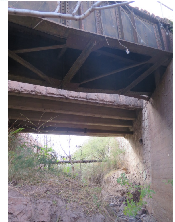
In the distance, Clifton sewer line (active), roadway bridge with abandoned pipe, original railroad bridge closest.
