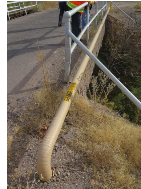
Southwest Gas line – West side of Bridge (Not attached to the bridge).
