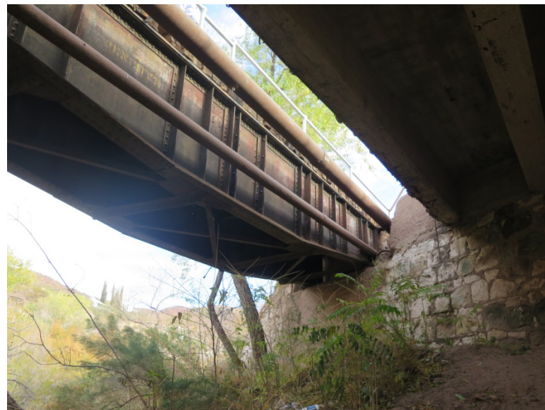
Two pipes between the bridges – lower is abandoned water line upper is active water main.
