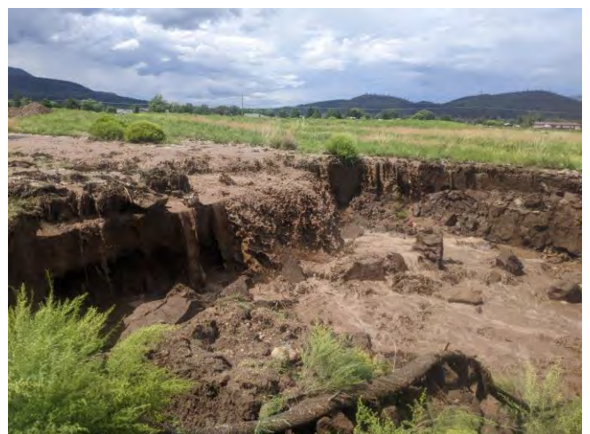
Severe Erosion Damage - Copeland Detention Facility
