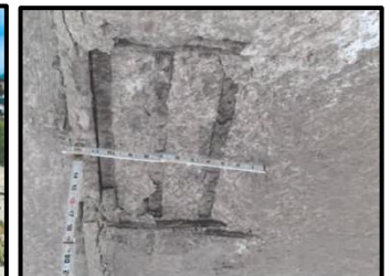
Large Spall in Soffit – Exposing Rebar
