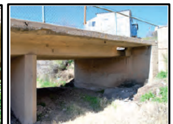
Scouring on piles
