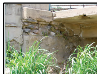
Abutment Wall Spall
