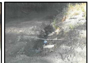
Erosion at the NW
