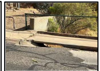
Pavement and Concrete Deterioration
