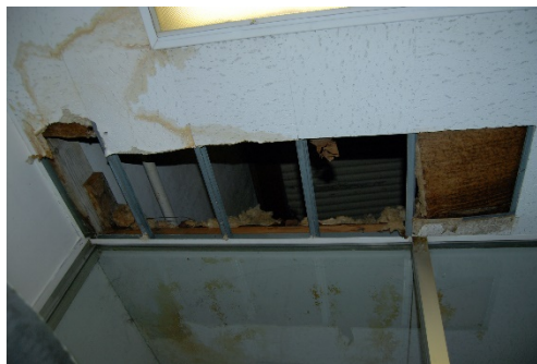
Figure 27: Water damage at suspended ceiling
