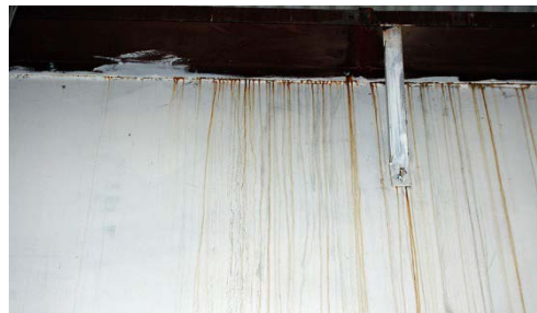
Figure 26: Water stains at interior surface of exterior concrete wall at connection to roof framing
