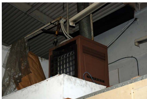
Figure 29: Gas-fired space heater.
