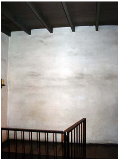
Figure 10: Soil at plaster finishes
