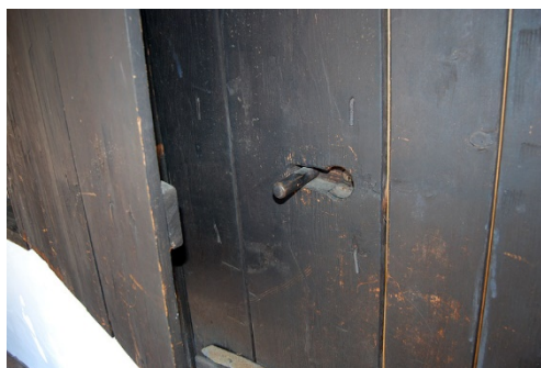
Figure 8: Wear at wood finishes
