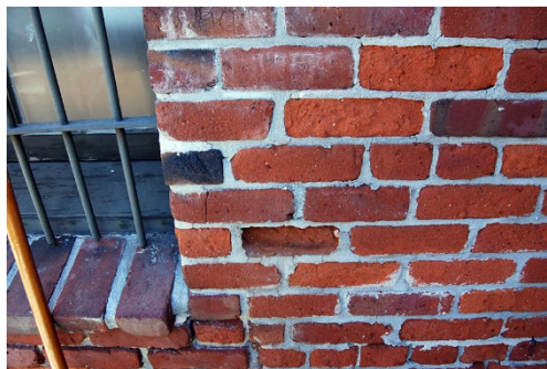
Figure 17: Eroded brick, mortar loss, poor mortar repointing profiles, with mismatched mortar composition (rear of Hellman/Quon building).
