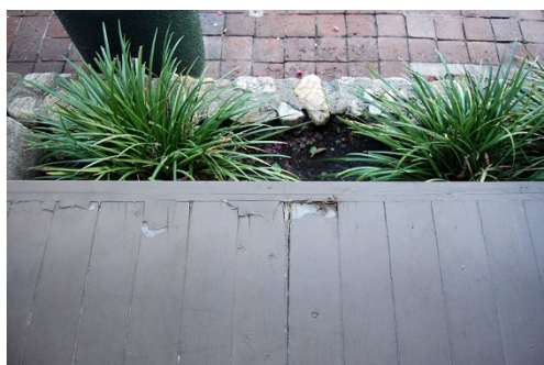
Figure 4: Damage at floor porch boards.
