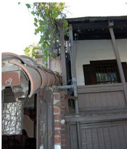
Figure 3: Meter and utility closet at northwest corner.
