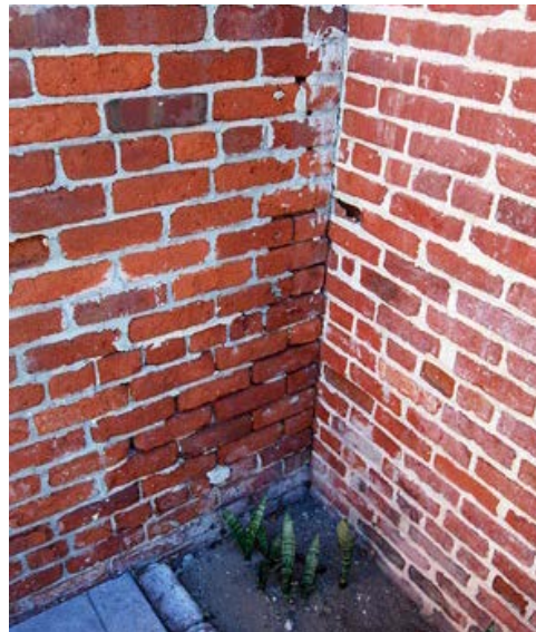
Figure 16: Eroded brick, mortar loss, poor mortar repointing profiles, with mismatched mortar composition (rear of Hellman/Quon building to left of inside corner).
