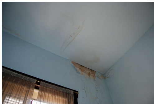
Figure 18: Water damage at ceiling and exterior wall.
