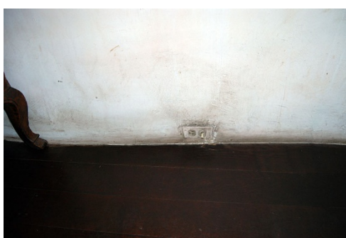
Figure 12: Damaged and unprotected power receptacle.
