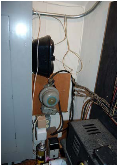
Figure 23: Equipment, clutter, dust, loose wiring, and aerosol can.
