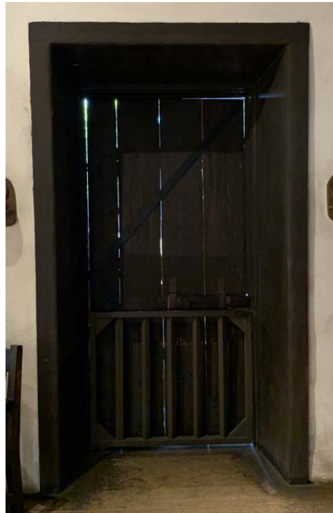
Figure 1: Detail of large gaps within and around exterior door in the Family Room.
