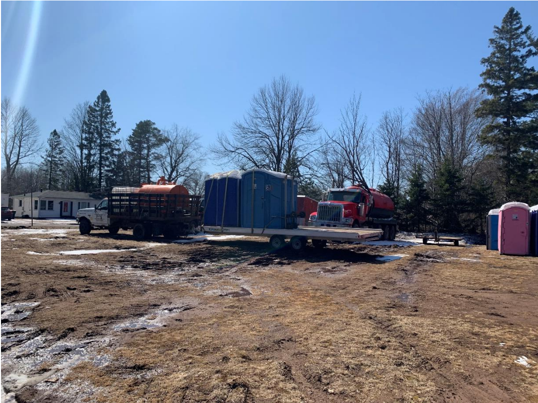
Photos of Tula Toilets Site (NW Corner of Hwy 2 and Walnut Street) Photos taken March 29, 2021
