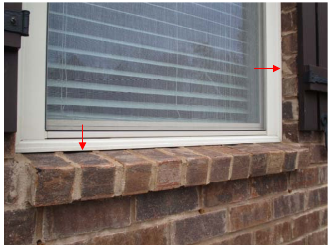
Caulking is needed around the perimeter of the second floor windows on the front of the home.
