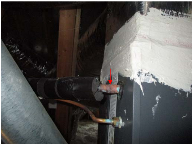
Additional insulation is needed around the refrigerant return line exiting each a/c evaporator coil in the attic to prevent condensation from dripping into the furnaces during the operation of the a/c units.
