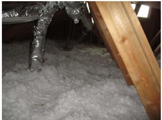
Re-distribute the blown-in insulation in the floor of the upper attic to provide consistent coverage which will help increase efficiency.
