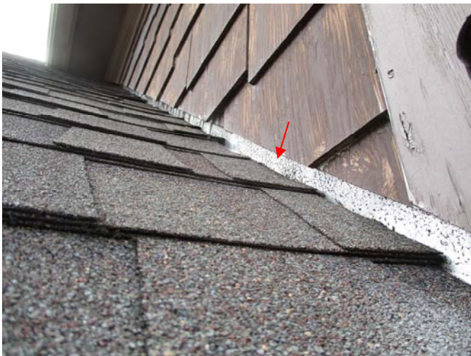
Counter flashing rather than step flashing was installed along the rooflines on the home.
