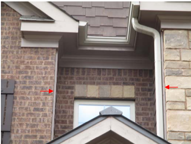
Caulking is needed along the vertical trim at all brick transitions on the home.
