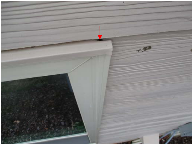
The header flashing is damaged at the upper corners of several windows in the siding portion of the home, which is a source of water entry behind the siding during rains.
