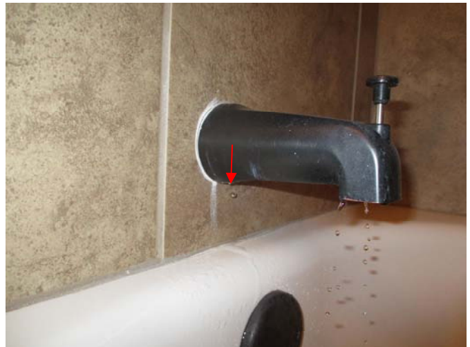
Water leaks out from the bottom of the tub faucet in the right, upstairs bedroom bathroom when the showerhead is engaged.
