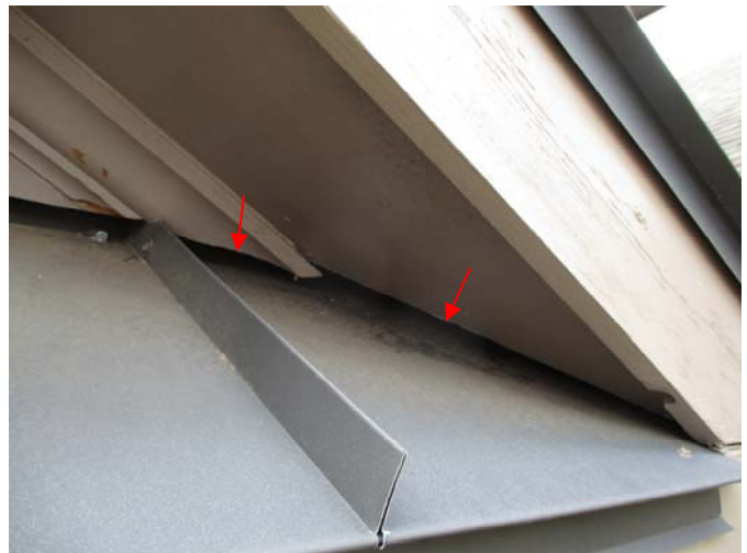
A qualified contractor should seal the construction gap under the soffit located below the right side of the gable on the front porch roof to help prevent future insect/rodent entry.
