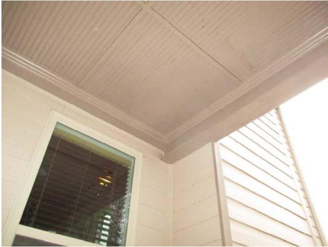
Active moisture stains were present on the siding, horizontal trim and paneling on the ceiling located below the left side of the roof above the covered patio on the back of the home.
