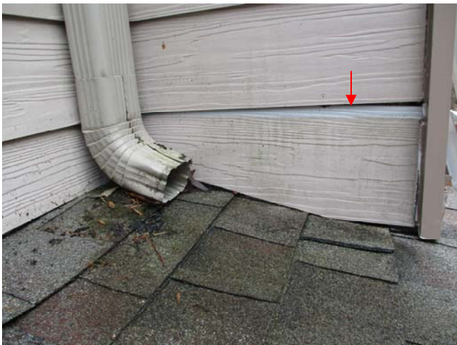
A qualified contractor should secure the displaced, lower piece of siding on the right side of the chimney chase located above the left, front corner of the roof above the covered patio on the back of the home.
