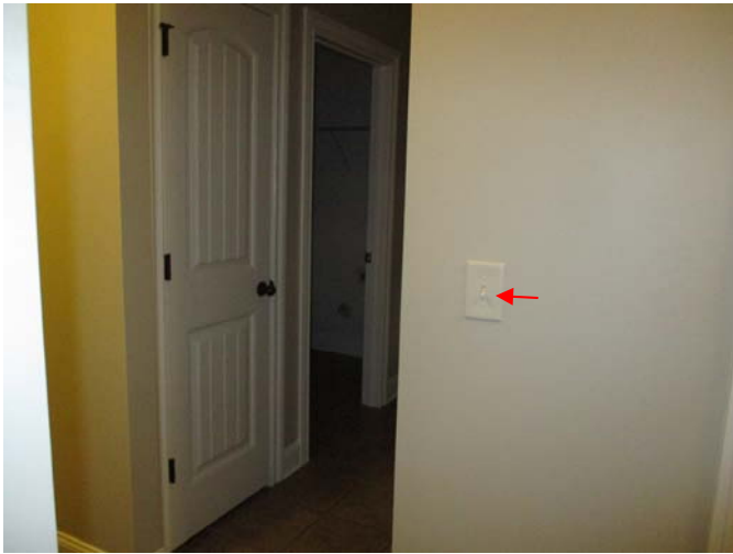
A licensed electrician or qualified contractor should replace the defective light switch located on the right side of the hallway leading to the laundry room.
