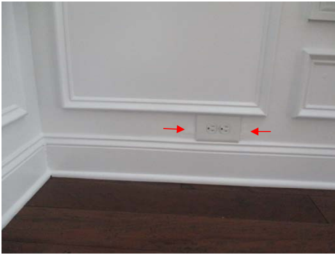
Swelling and moisture stains were present on the wainscoting located around the outlet in the right, front corner of the formal dining room.
