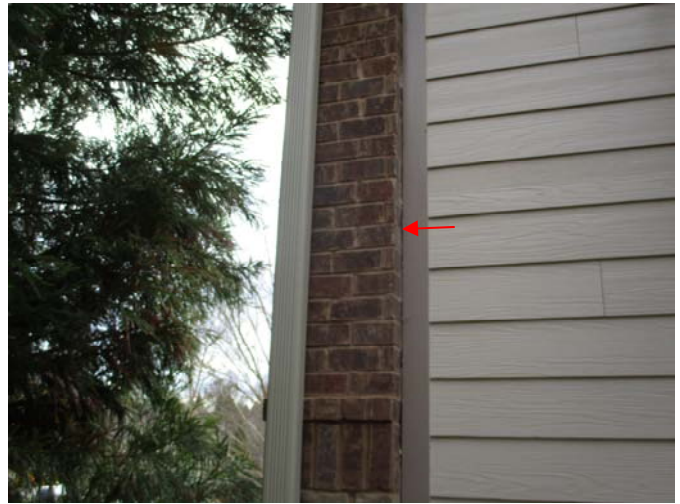
Caulking is needed along the vertical trim at all brick transitions on the home.
