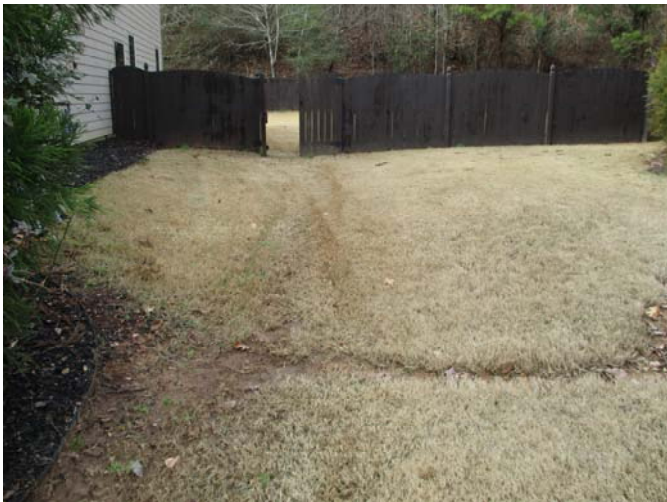
The sod/soil along the swale on the right side of the home was very soft and saturated at the time of the inspection.
