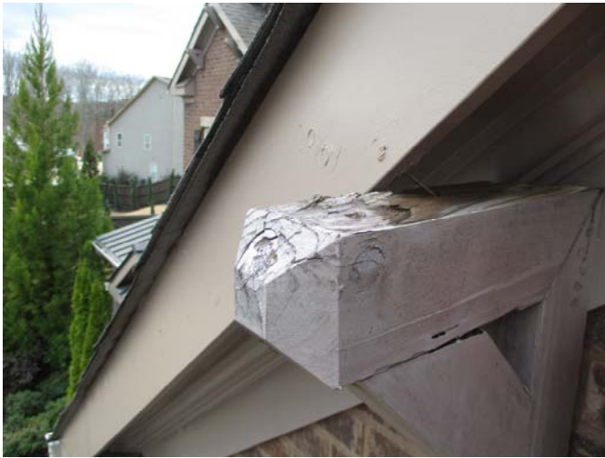
Updated paint is needed on the decorative beams located along the gables on the front of the home.
