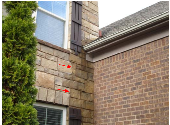
Active moisture stains were present on the stone cladding below the roof termination located above the right, front corner of the formal dining room.
