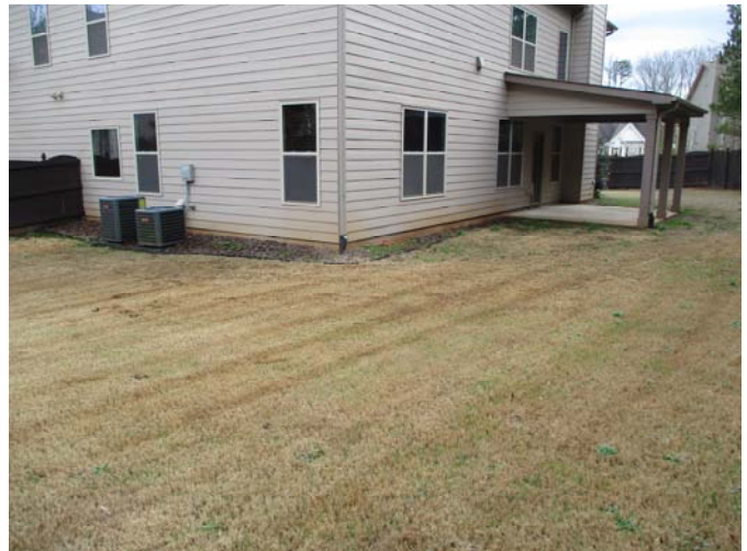
The sod/soil along the swale around the back of the home was very soft and saturated at the time of the inspection.
