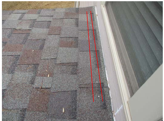
Several exposed nail heads were present in the upper rows of shingles on the roof located above the covered patio on the back of the home.
