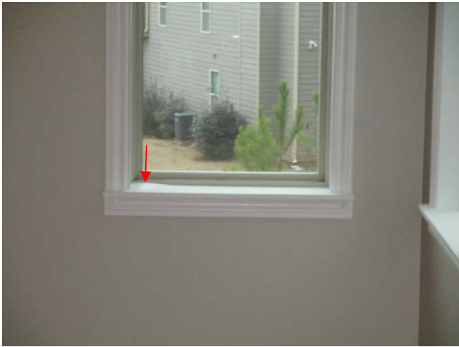
The interior sill is swollen below the left side of the upper, right window in the left wall of the family room (. . .)
