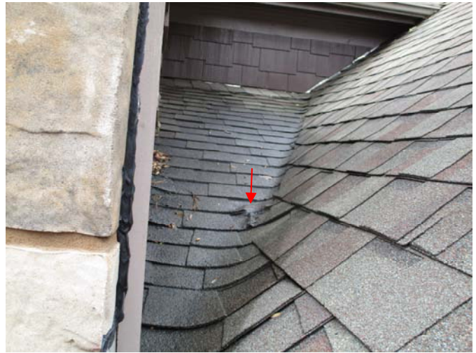
The shingles located at the bottom of the roof valley outside the right wall of the front, center bedroom are raised and have been sealed with roofing tar.
