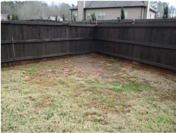
Standing water was present inside the left, front corner of the fence on the left side of the home at the time of the inspection.
