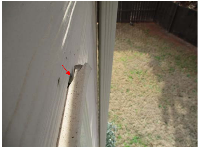
The header flashing is damaged at the upper corners of several windows in the siding portion of the home, which is a source of water entry behind the siding during rains.
