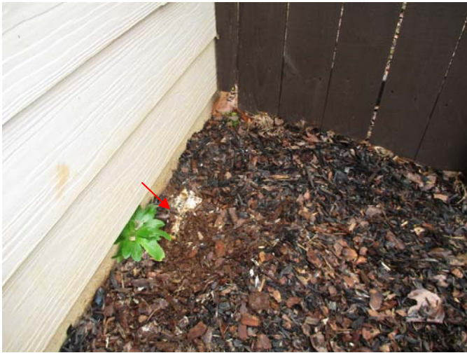
The a/c condensate drainlines terminate along the foundation in front of the fence on the right side of the home.
