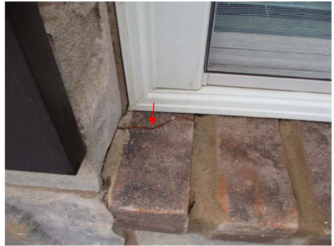
A qualified contractor should seal the cracked brick below the left side of the windows in the front, center bedroom to help prevent future moisture entry.
