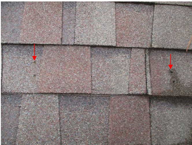
Unsealed toe board nail holes were present in the shingles above some of the gutters around the perimeter of the home.
