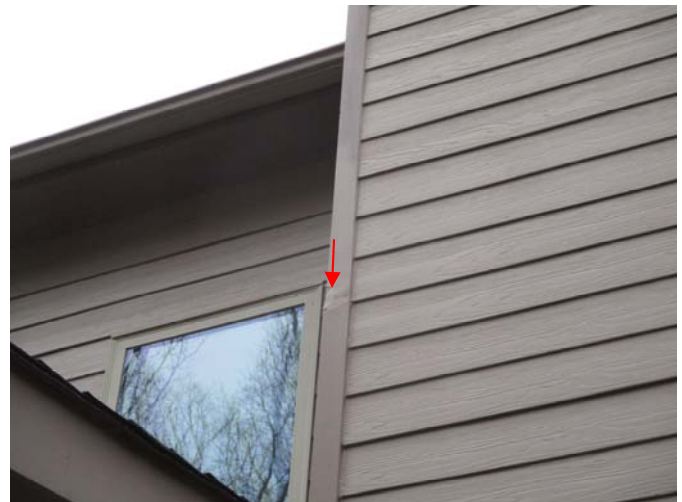
Moisture damage was present at the vertical trim midway-down the right side of the chimney chase.
