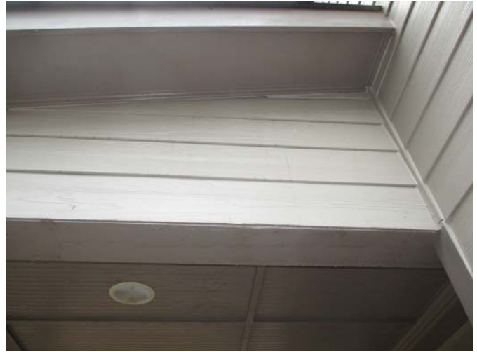
Active moisture stains were present on the siding and horizontal trim on the ceiling located below the left side of the roof above the covered patio on the back of the home.
