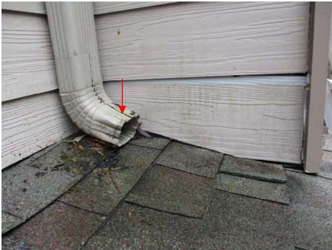
The roof flashing is torn behind the vertical trim on the right side of the chimney chase located above the left, front corner of the covered patio on the back of the home, which is allowing moisture entry under the shingles during rains.
