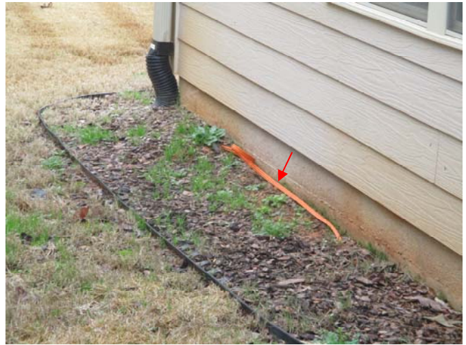
Please consult with the homeowner about the buried/exposed, orange wiring running along the foundation around the rear portion of the home.
