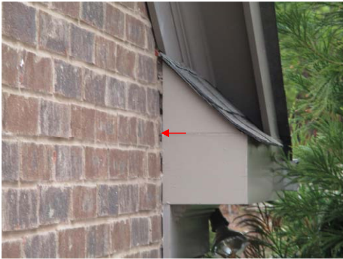
Caulking is needed along the sides of the gable returns on the front of the home.
