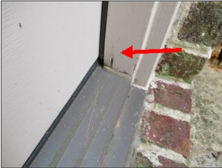
Minor wood damage at basement door
