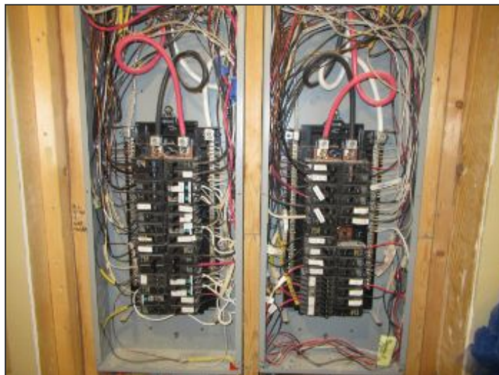
Interior view of main panels
