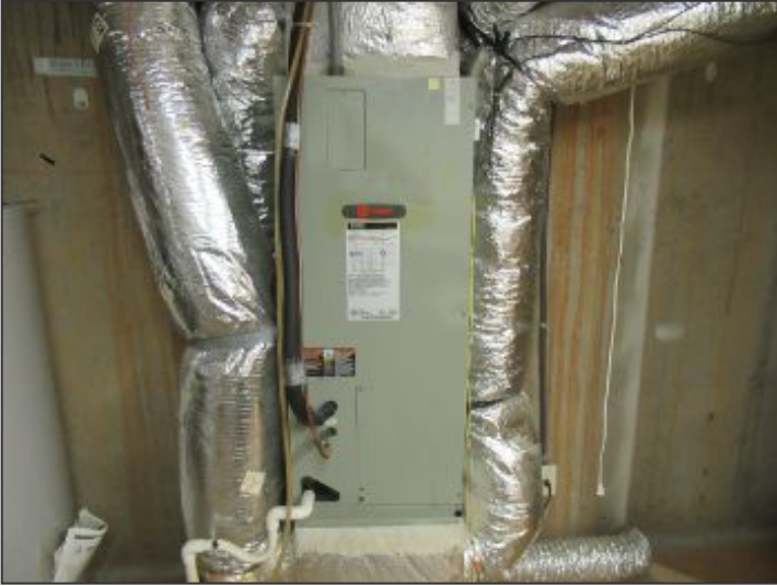
Basement air handler located in basement
