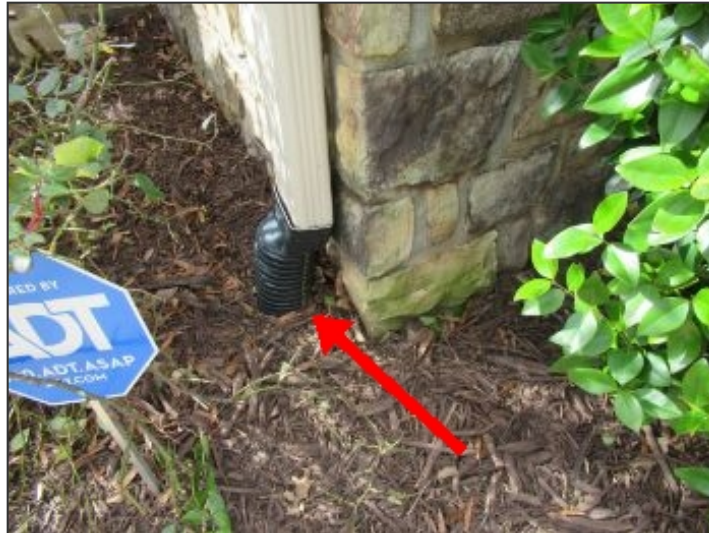
Downspouts piped underground for improved drainage
