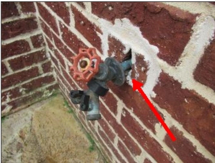
Basement door hose bib projects too far outside wall
