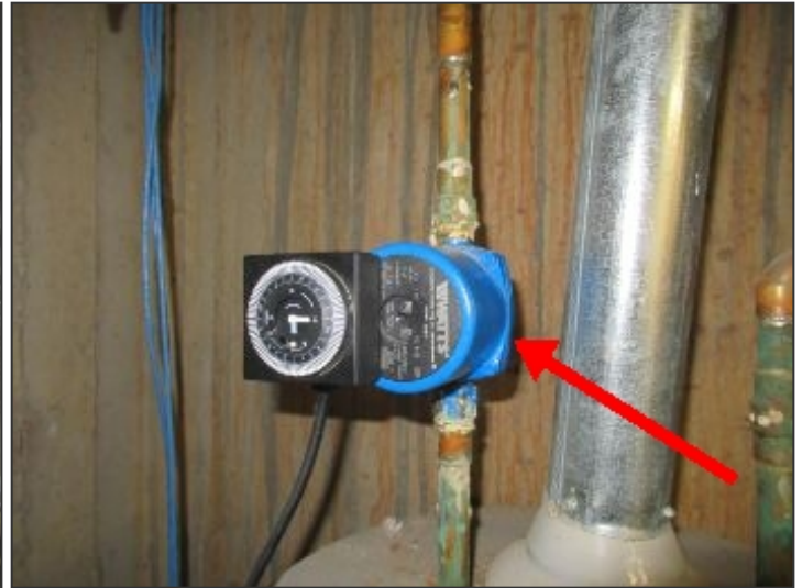
Recirculating pump at water heater
