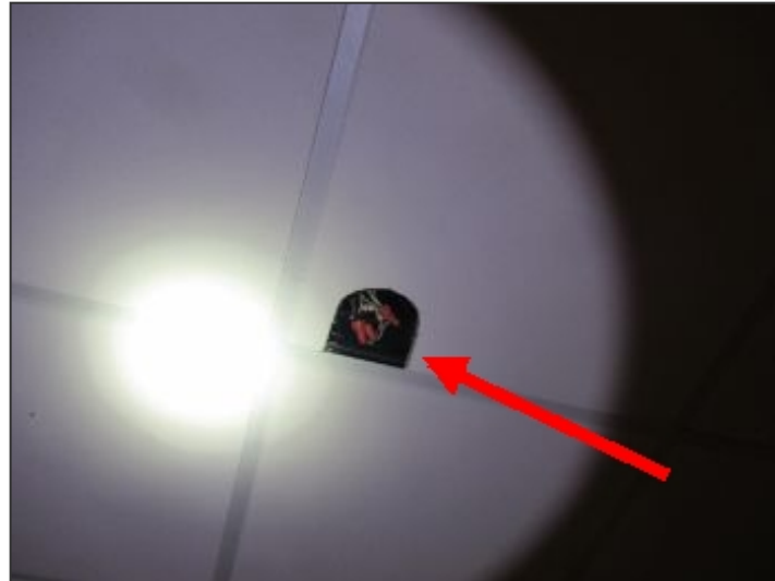
Missing light at basement ceiling
