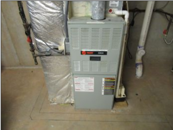
First floor furnace located in basement
