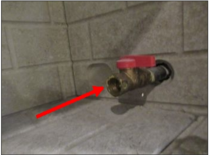
Open gas line at basement fireplace
