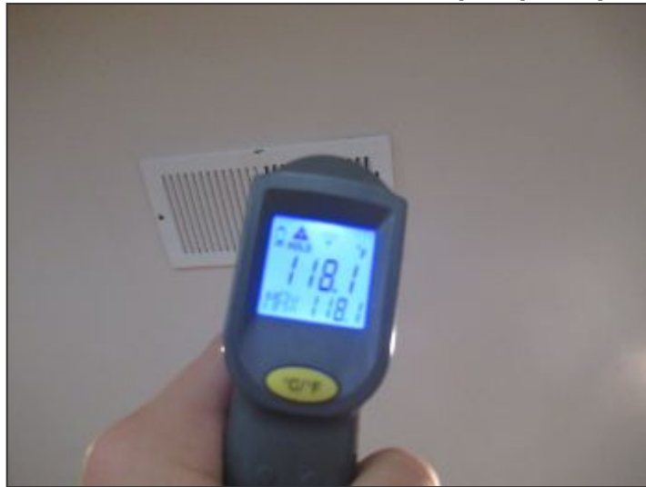
Heat pump / strips temp normal at 118 degrees
