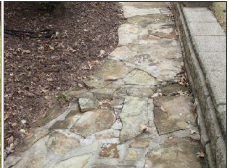
Damaged stones at right yard sidewalk
