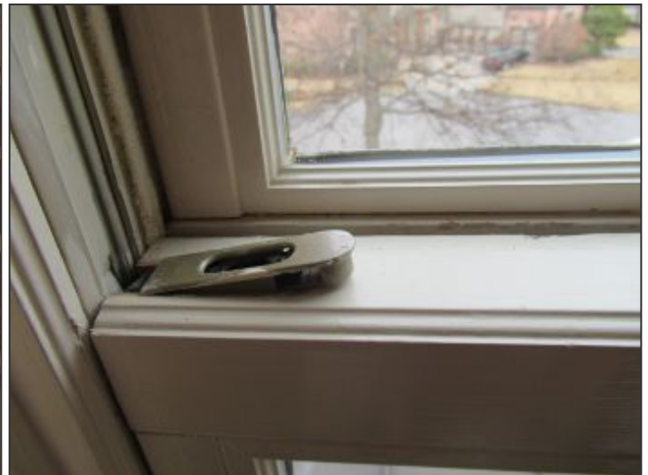
Broken window tilt latch
