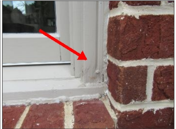
Minor trim rot at rear kitchen keeping room window
