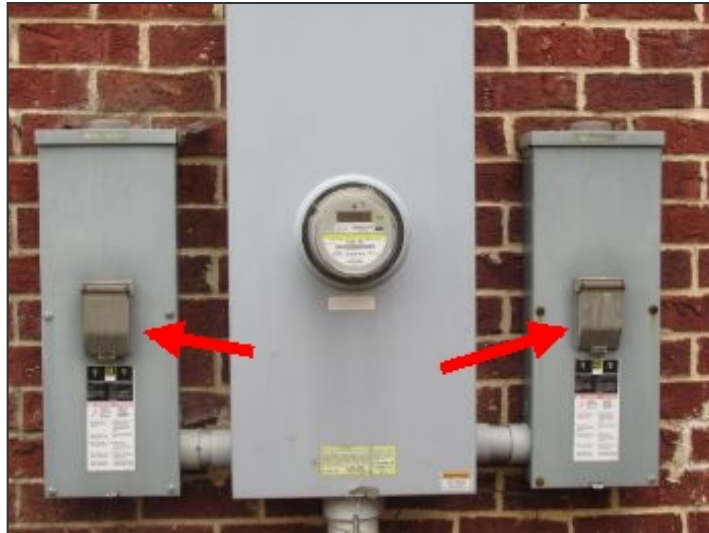
Main breakers located outside
