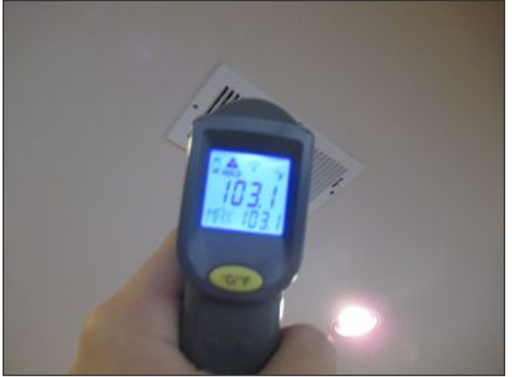
Heat pump temp normal at 103 degrees
