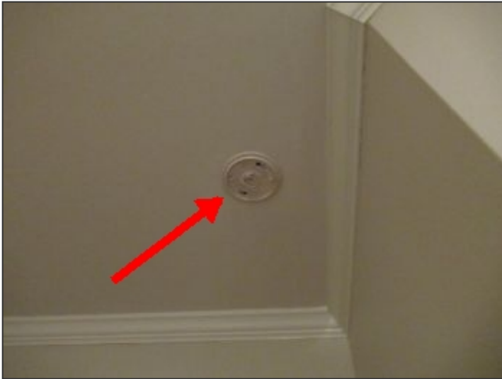
Smoke detector removed in basement
