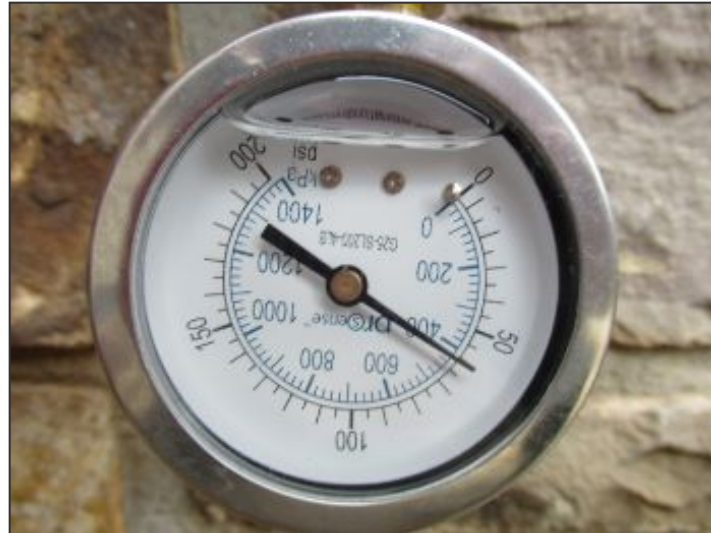
Normal water pressure at 60 PSI
