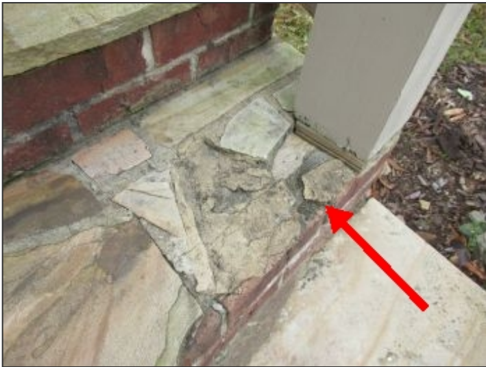
Damaged stones at front porch steps
