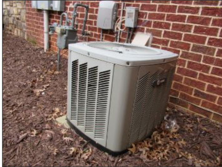
First floor AC unit
