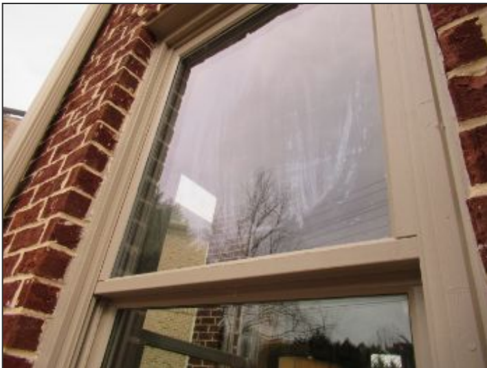
Defective window at rear kitchen keeping room
