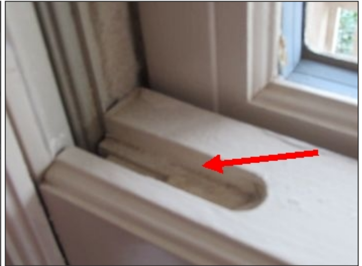
Missing tilt latch
