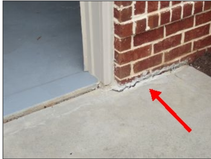
Driveway has dropped slightly at garage
