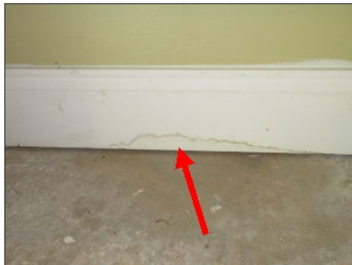
Water stain at baseboard below main water cut off
