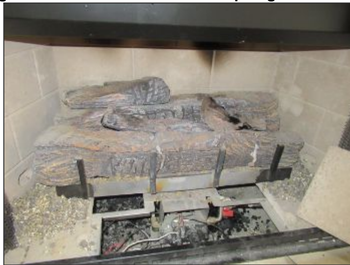
Unable to light kitchen keeping room fireplace
