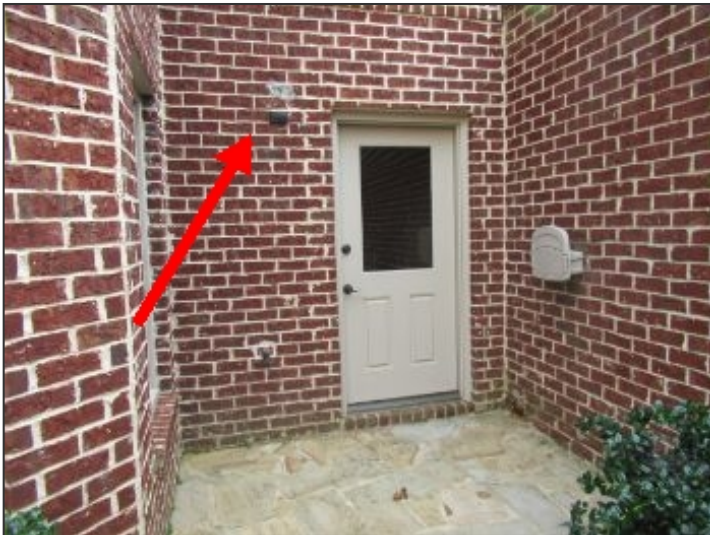
No exterior light above basement entry door
