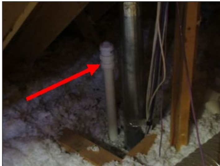
Studor vent above master closet laundry room
