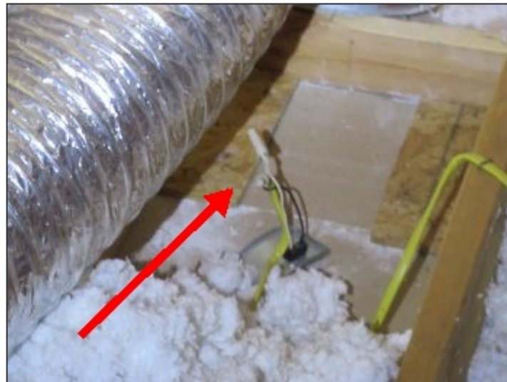
Wiring splice in attic above master shower
