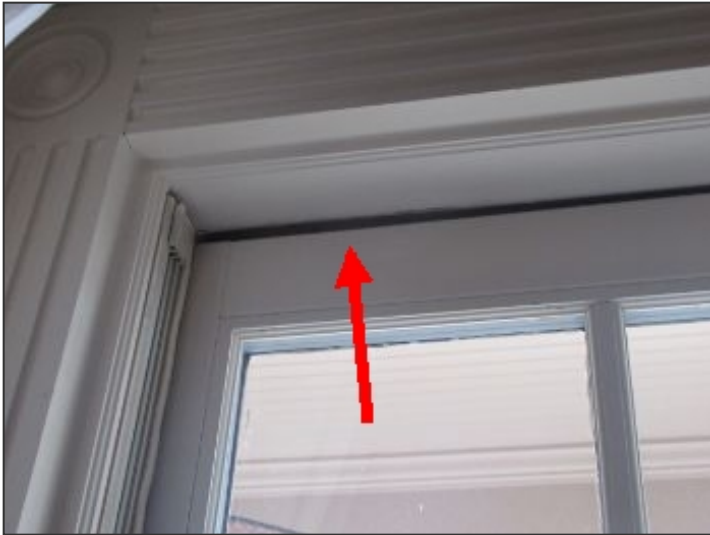
Dining room window not fully closed
