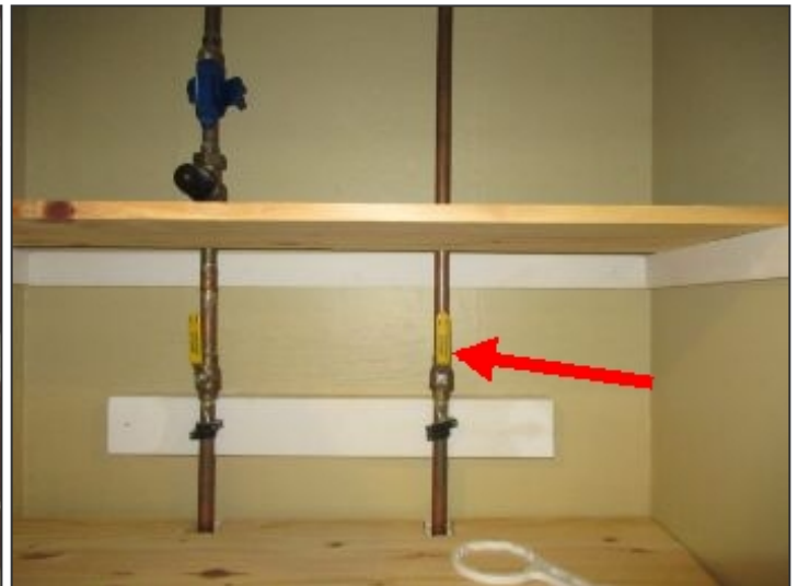
Main water cut off located in basement
