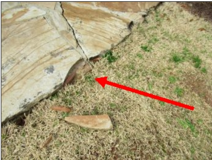
Damaged stones at front sidewalk
