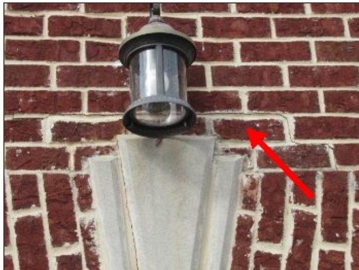
Small crack at brick above garage doorway
