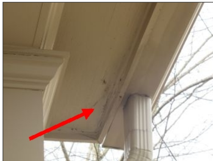
Damaged wood soffit at front porch roof
