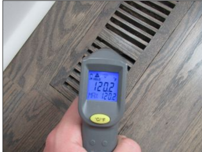
First floor furnace temp normal at 120 degrees
