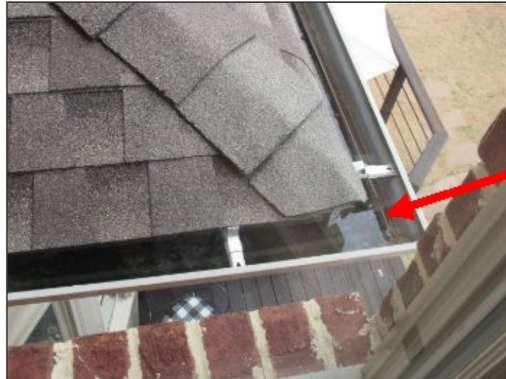
Gutter holding water above family room windows
