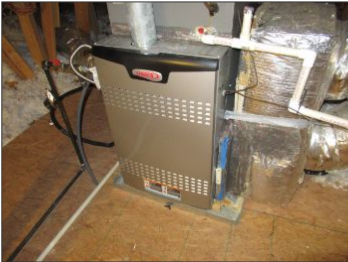
Second floor furnace located in attic
