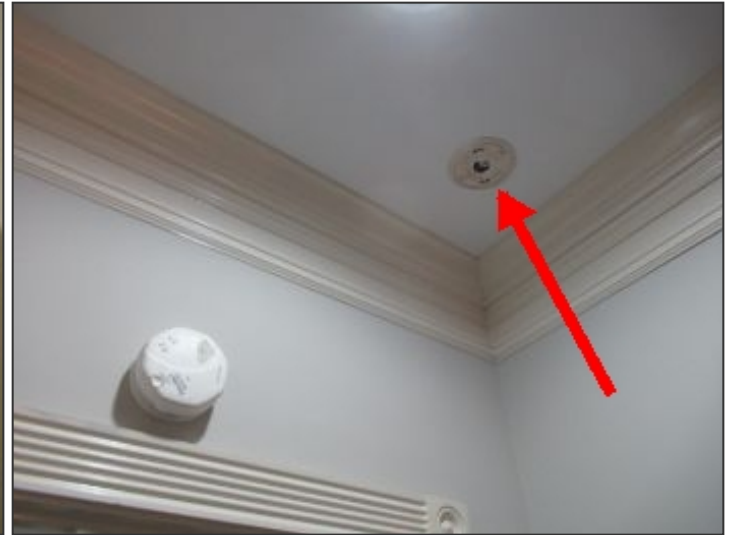
Smoke detector removed near master bedroom
