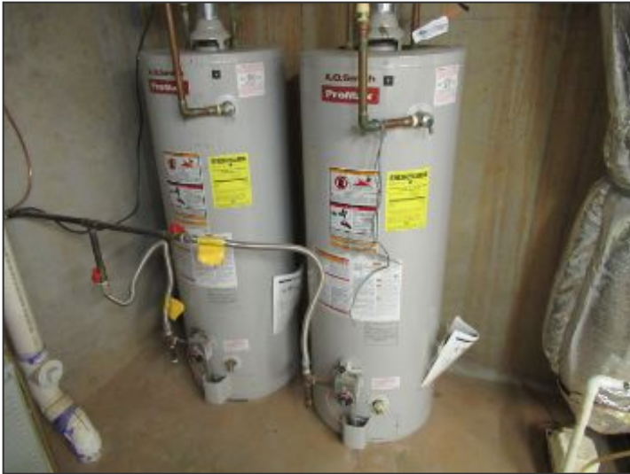
Water heaters located in basement
