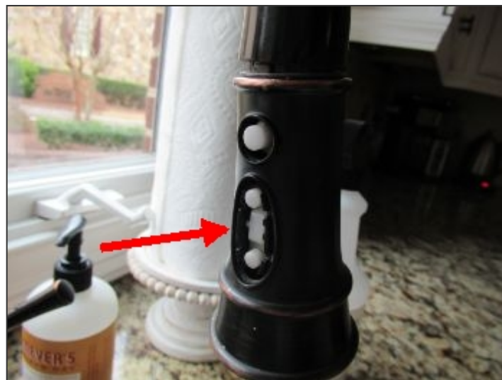
Diverter buttons missing
