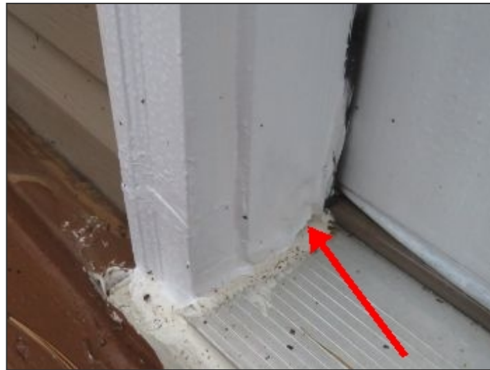
Damaged trim and wood filler repair at deck door jamb
