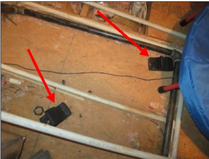
Rodent traps in attic
