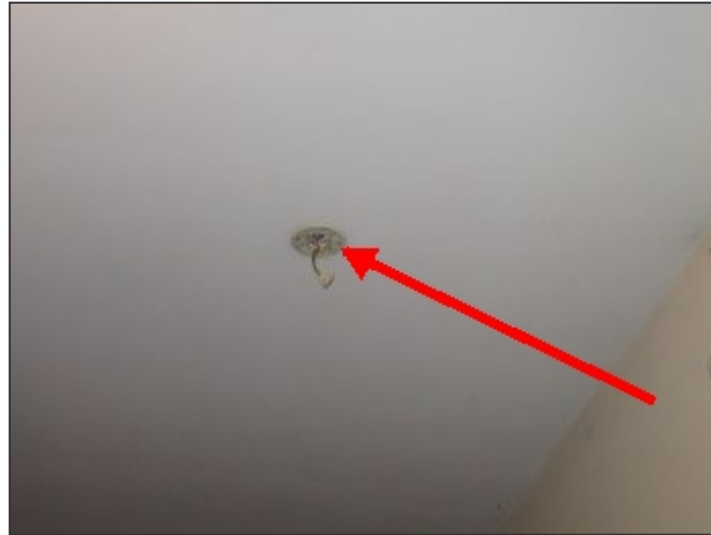
Garage smoke detector removed
