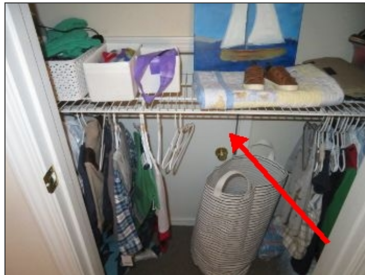
Unable to access partial attic space - entry door obstructed by shelving
