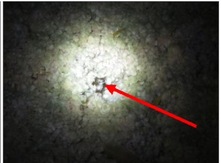
Rodent tunnels in attic insulation
