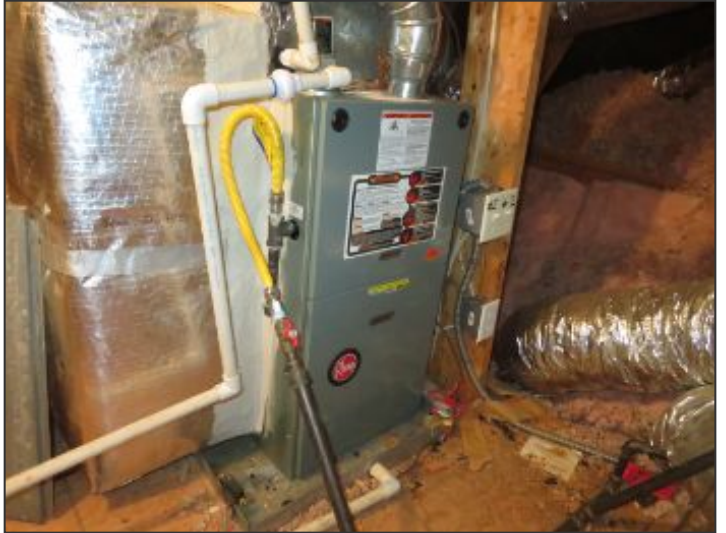
First floor gas furnace in attic
