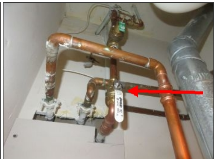
Main water cutoff above water heater
