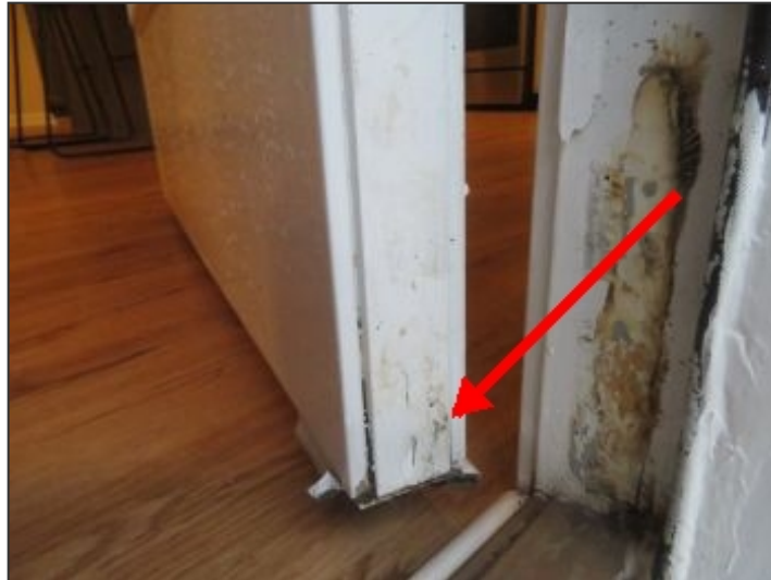
Minor damaged wood at deck entry door
