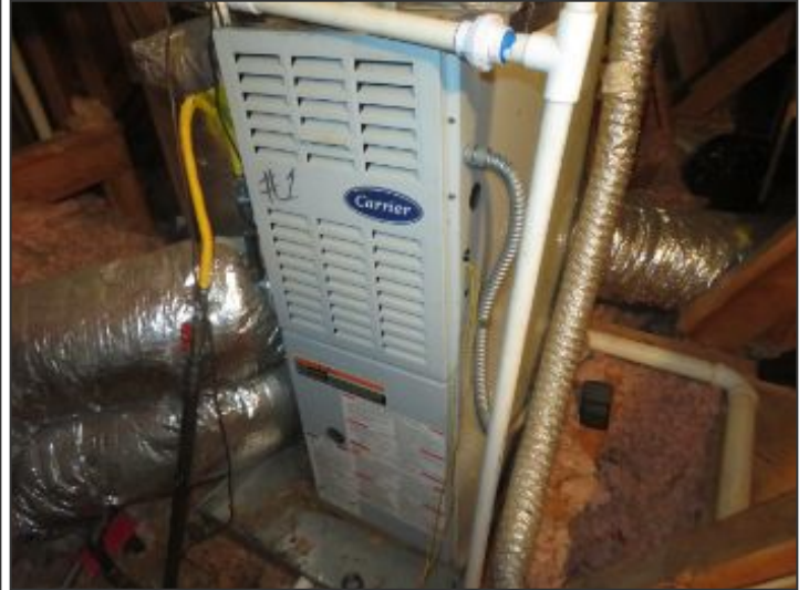
Second floor gas furnace in attic
