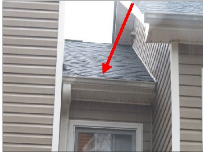
Gutter improperly sloped at rear roof near chimney
