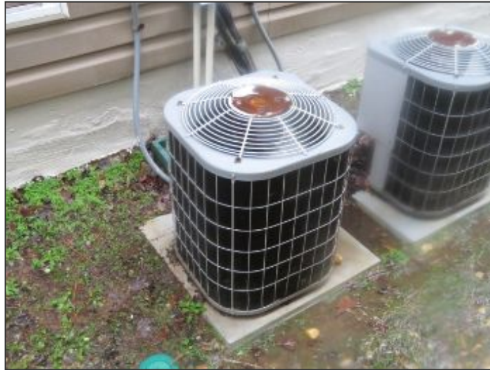
First floor AC unit
