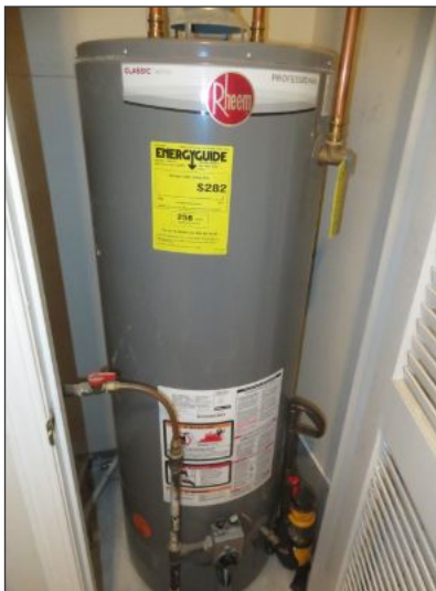
Gas water heater in laundry room
