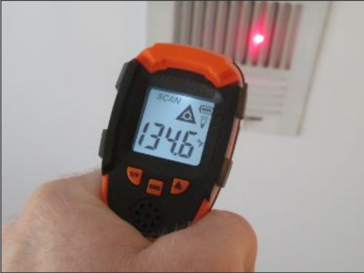
Gas furnace heating normally - 134 degrees
