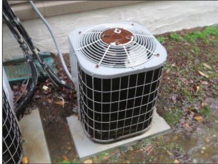
Second floor AC unit
