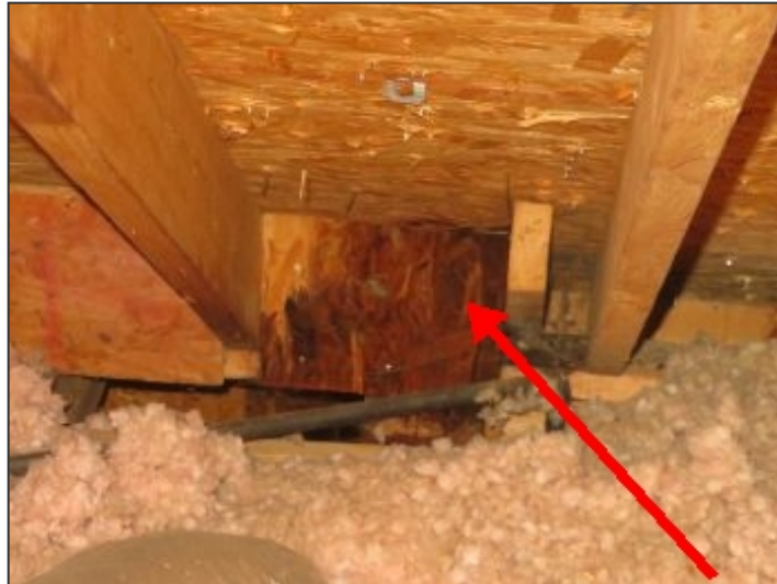
Active leak in attic at chimney - wet stains present
