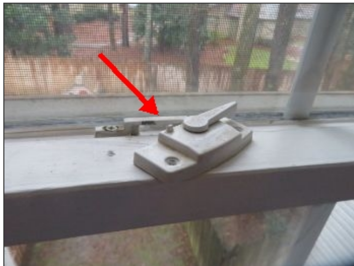
Loose lock at rear right guest bedroom window
