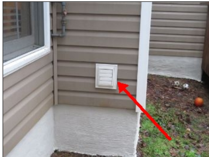
Improper fresh air vent cover at chimney
