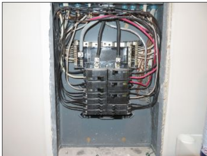
Interior view of main panel
