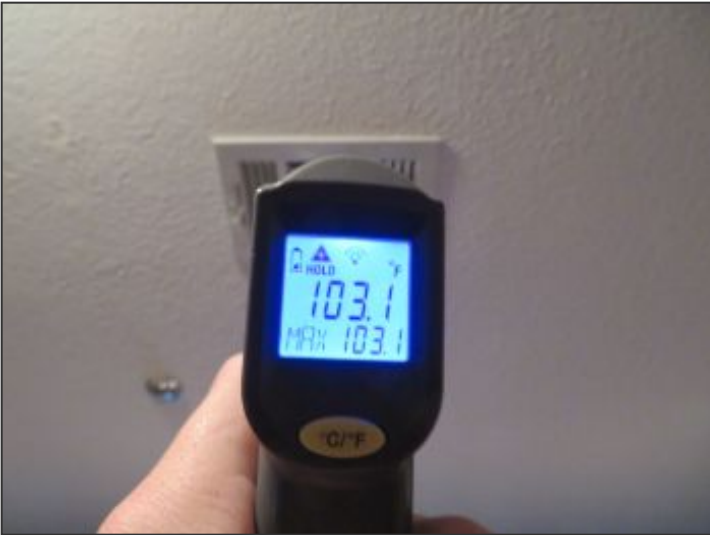
Heat pump temp normal at 103 degrees
