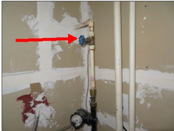
Main water cut off located near water heater
