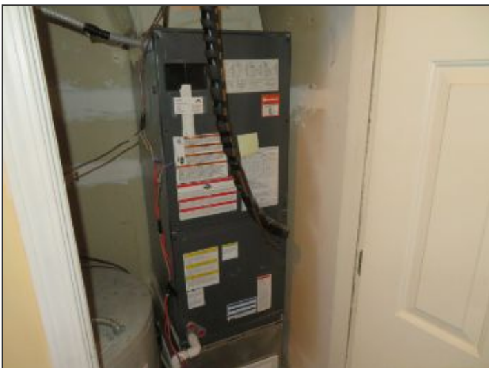
Air handler located in hall closet
