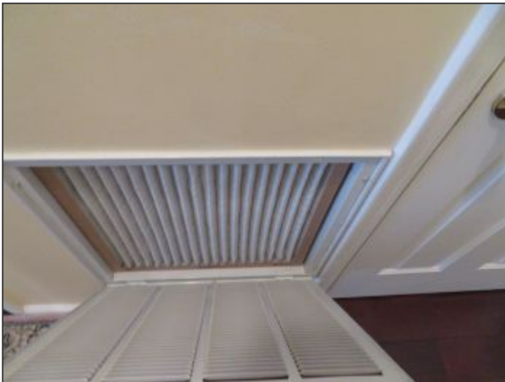
Location of wall filter
