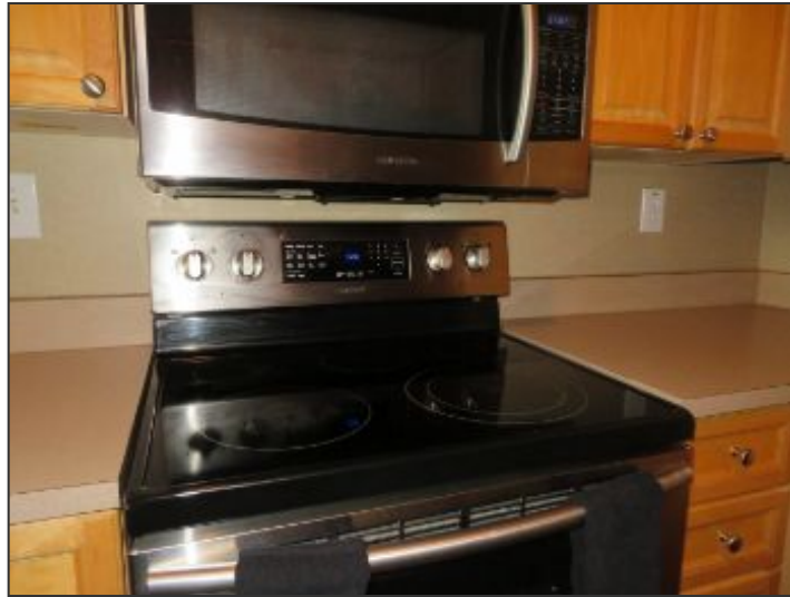
Microwave clearance too low
