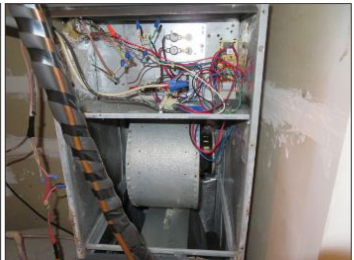
Interior view of air handler
