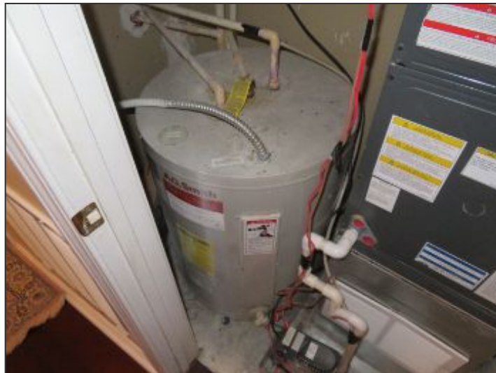
Water heater located in hall closet
