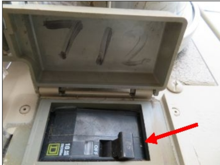
Main electrical cut off at exterior
