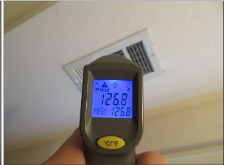
Heat pump / strips temp normal at 127 degrees
