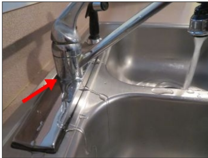
Faucet handle leaking when tested
