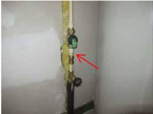
Photo 49-1 Leaking near main shut off.
