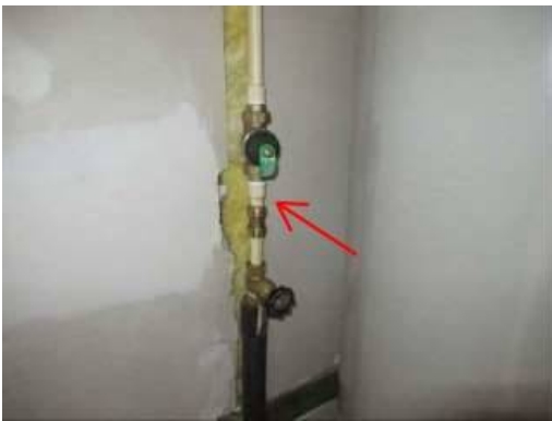
Photo 49-1 Leaking near main shut off.
