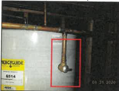
Missing bleeder valve noted.
