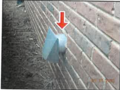
Vent hood found loose and not sealed to the wall surface.
