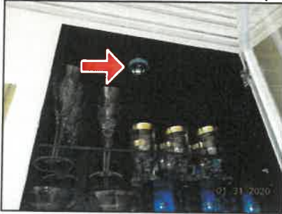
Inoperable light noted.
