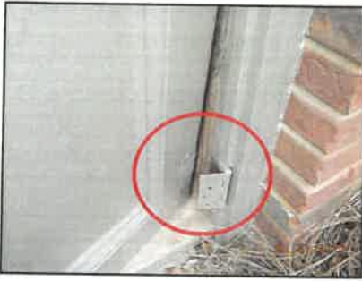
Loose hinge noted.
