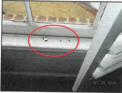
Broken/missing shutter magnets noted.
