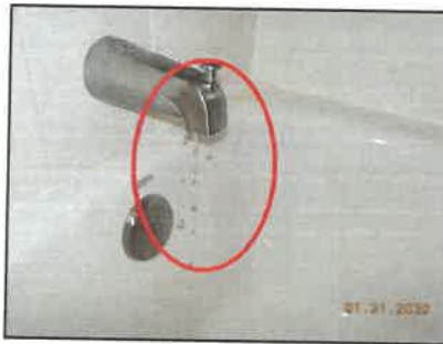
Shower diverter does not seal completely when engaged.
