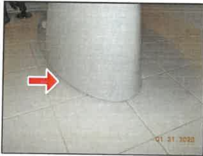
Toilet should be sealed between the base and floor
