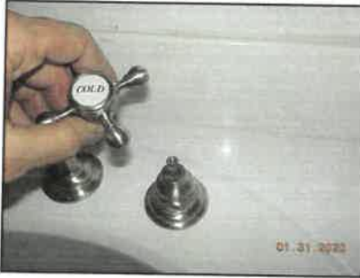
Loose faucet valve handles noted.
