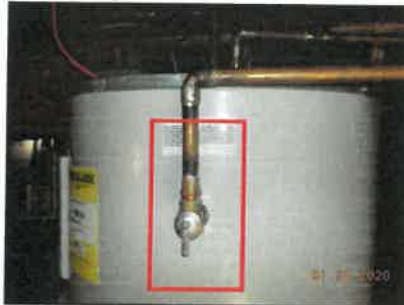
Missing bleeder valve noted.
