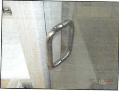
Loose shower door handle noted.
