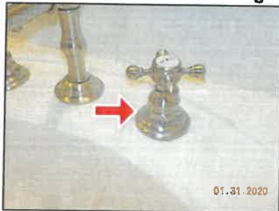
Loose faucet valves noted.
