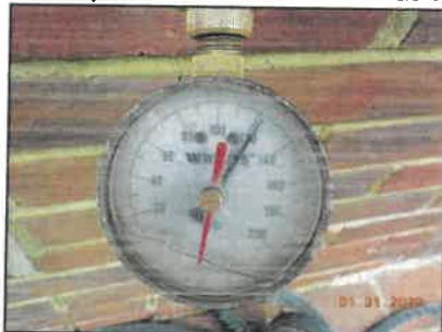
The water pressure was recorded at 120+ PSI
