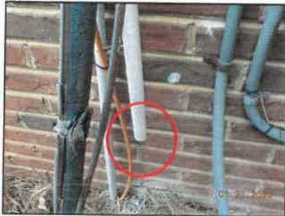
The condensation drain line terminates next to the building.
