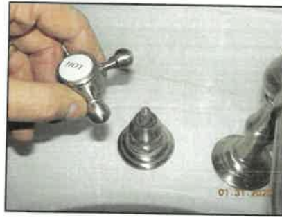
Loose faucet valve handles noted.
