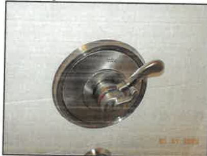
Reversed hot and cold plumbing noted at the tub/shower valve.
