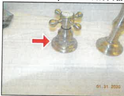
Loose faucet valves noted.
