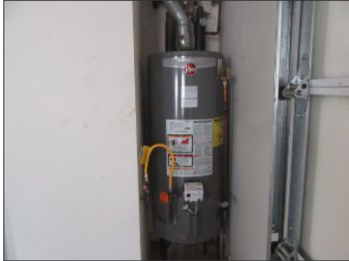
Water heater in the garage
