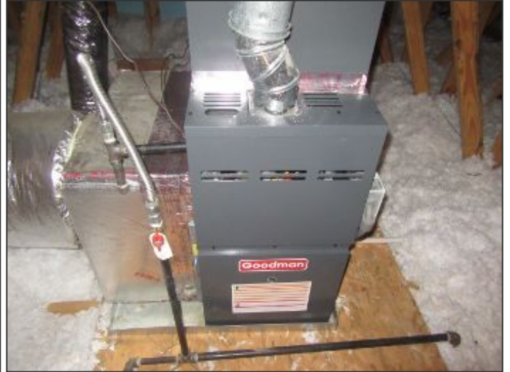
Furnace in the attic
