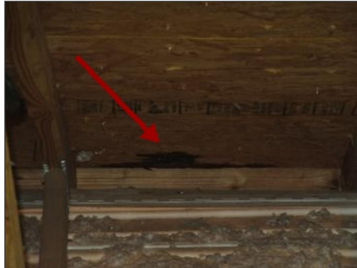
Old stain in the attic above the front porch roof
