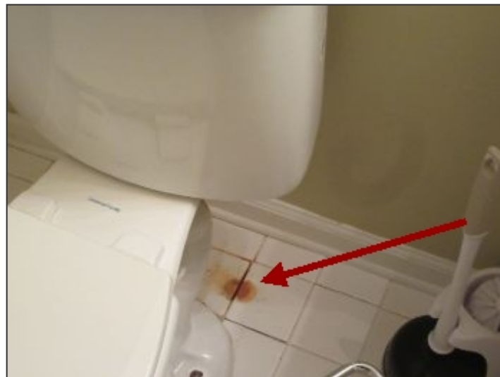
Guest bathroom toilet leaks at the bolts
