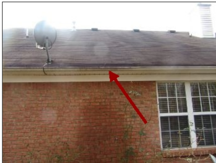
Gutter full of debris and overflowing at the rear roof
