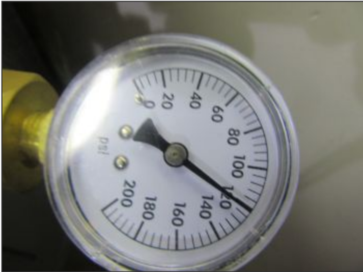
Water pressure too high at 120 psi
