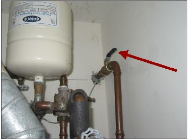
Main water cut off in the garage
