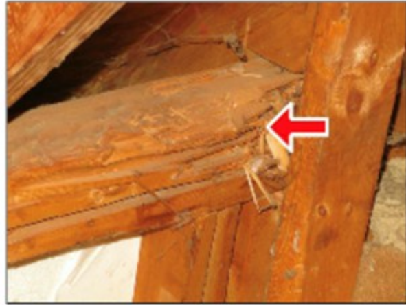
5.0(2) ROOF FRAMING (Picture 1) Damaged framing
