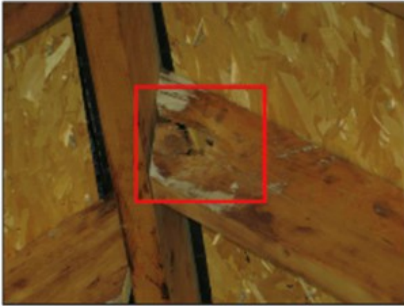
5.0(1) ROOF FRAMING (Picture 1) Hole in frame member
