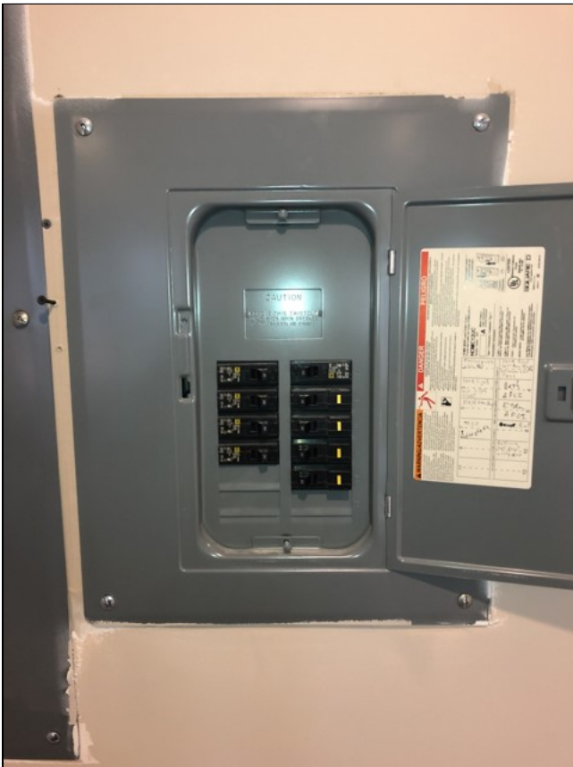
9.2 (3) Square D 125 amp electrical electrical subpanel.
