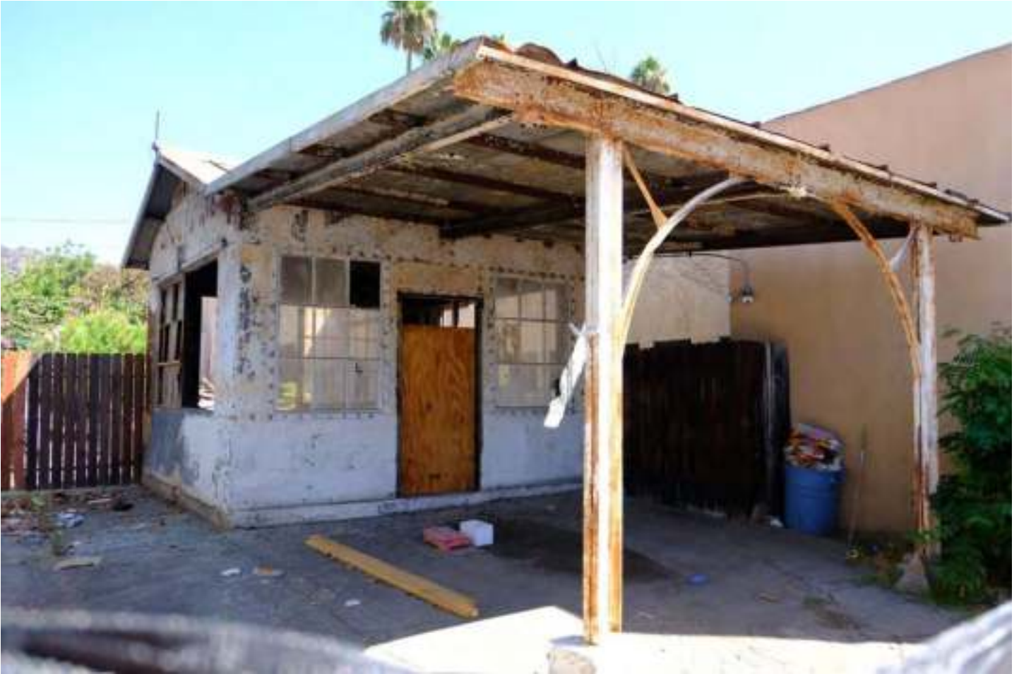
Jay Risk Standard Oil Co. Service Station. View northeast. Photographed after the owner started to disassemble the building. (Sullivan 2022)
