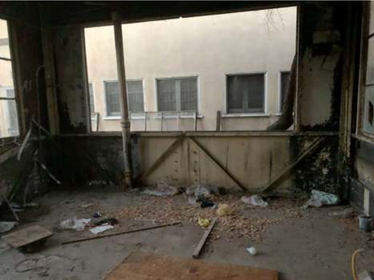
Jay Risk Standard Oil Co. Service Station. Interior. View east. Photographed after the owner started to disassemble the building. (Sullivan 2022)
